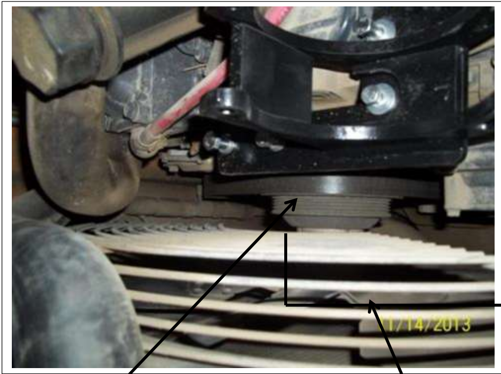
Compressor will drive off of this 4 groove pulley.
